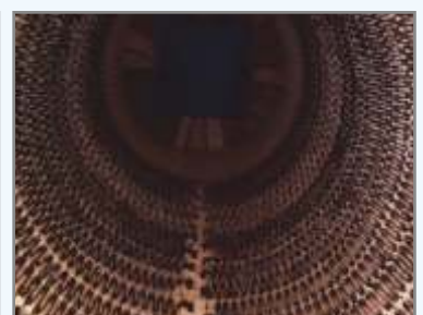
350 KW PYROLYTIC REACTOR FURNACE FOR FLUOROCARBONS
